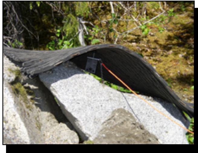
Figure 7—A rubber doormat helps contain flying rock and holds the BMS Micro-Blaster in place.
